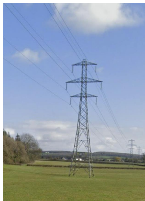
Figure 6-1: 132 kV double circuit OHL on steel lattice tower
